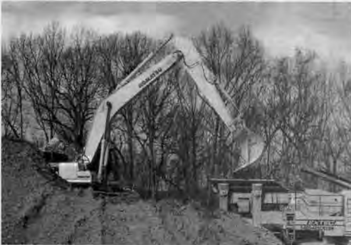
For the city's new water plant, site work is currently being performed and the infrastructure, pipe, foundations and footings are being installed. It should be completed within two years.
